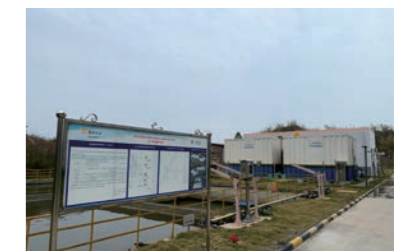
The zero wastewater discharge project in Luchuan Cement
